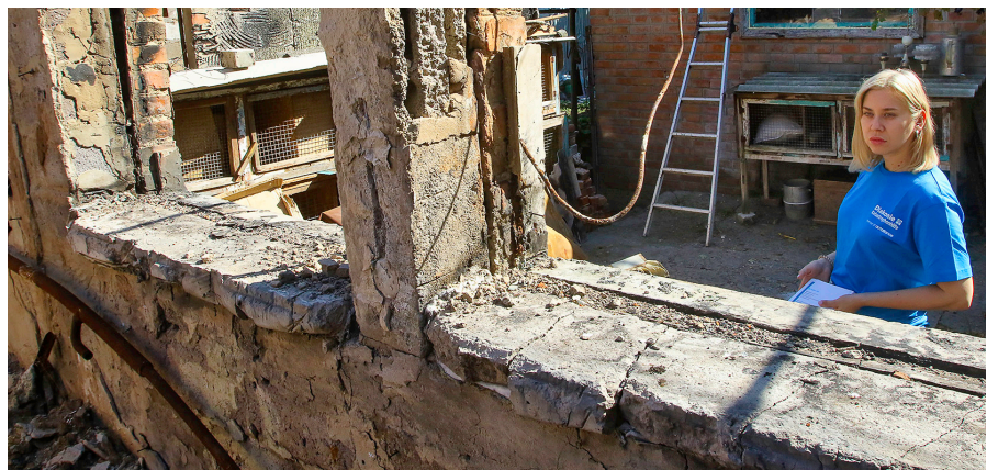
An employee of Diakonie Katastrophenhilfe inspects a destroyed living space in Ukraine. Our partner's teams of craftspeople are working hard to repair thousands of homes.
